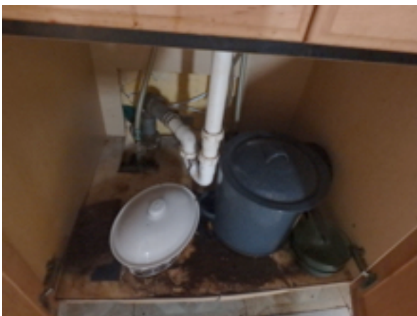
Typical poor older plumbing
