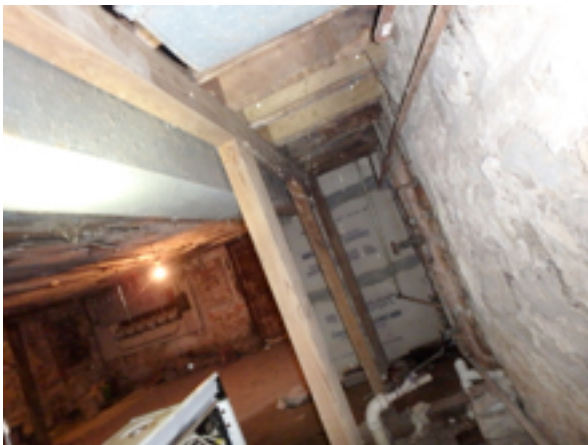
Poor joist tie-ins
