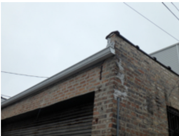
Typical wall erosion signs
