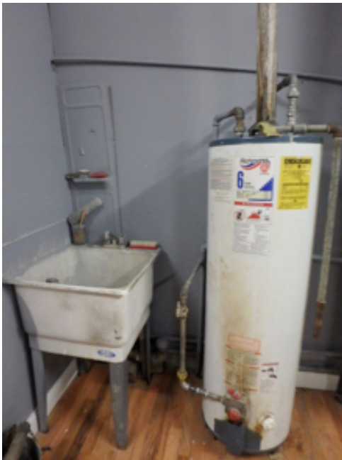
Flame roll out signs at storefront water heater
