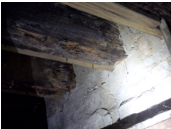
Another view of termite type damage at joists
