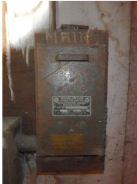
Old main disconnect
