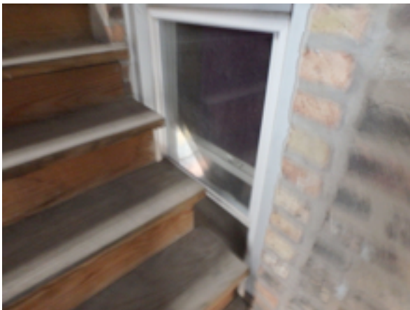
No guardrail along window
