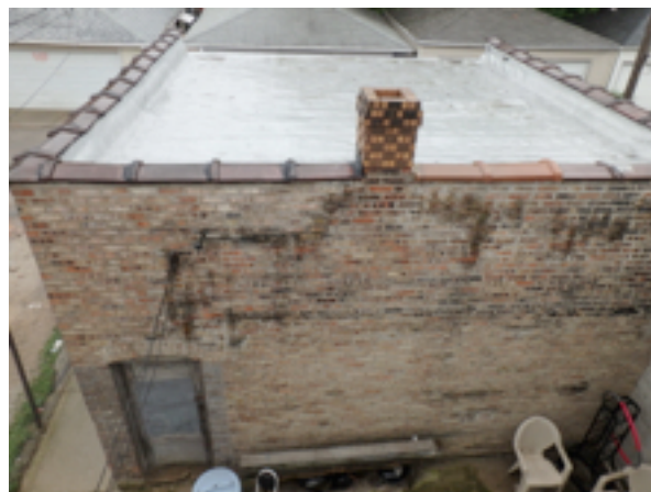
Wall erosion signs due to open chimney
