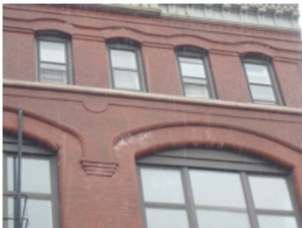
The white color on brick is water Saturation into the wall
