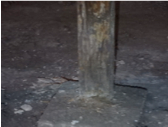
Typical mid span post rotted out at Floor level, all need replacement
