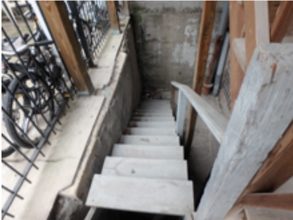
Stairway not fully compliant
