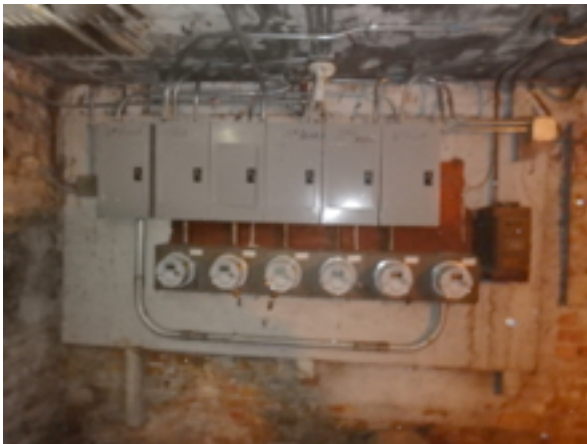
Electrical meter gang in basement
