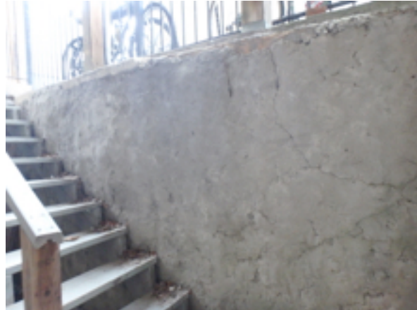
Retaining wall bulging inward
