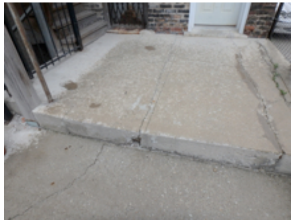
Multiple full length pad cracks
