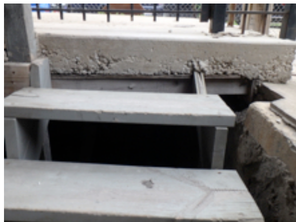
Poor stringer attachment
