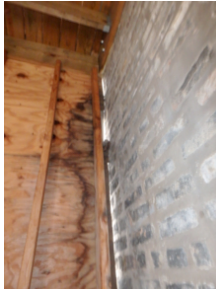
Water damage from downspout along the Exterior of the wall
