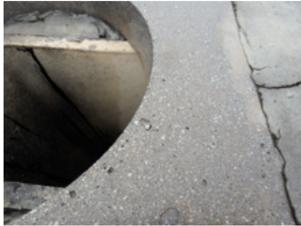
Typical poor open joints at top of chimney
