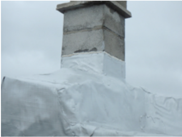
Typical poor installation, no term bar
