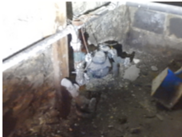
Water main in basement
