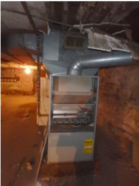
Storefront furnace in basement
