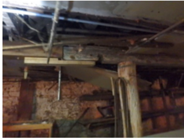
Poor beam and joist conditions
