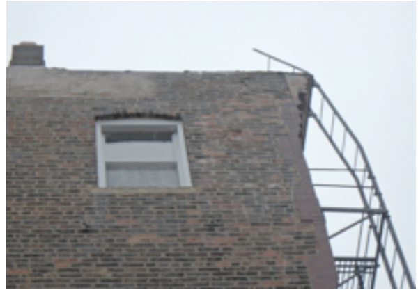
Typical erosion at front corners
