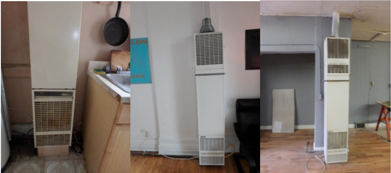
Typical mid-age Williams space heaters, better condition but still not ideal
