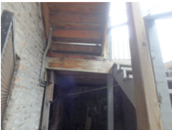
Lots of water saturation at wood
