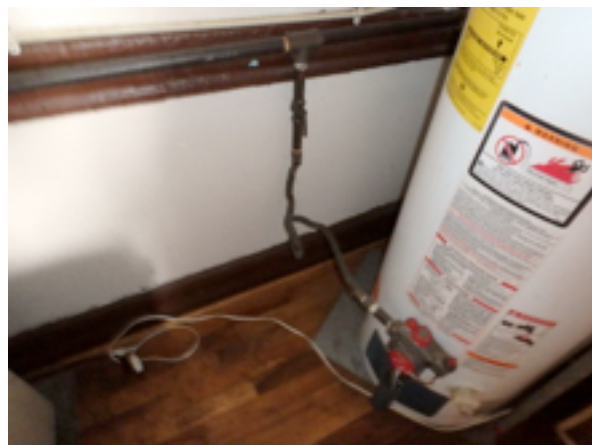
Poor gas connection at water tank
