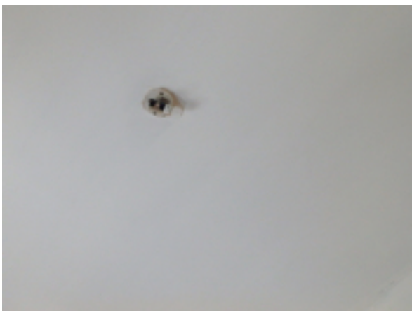
Typical damaged smoke detector
