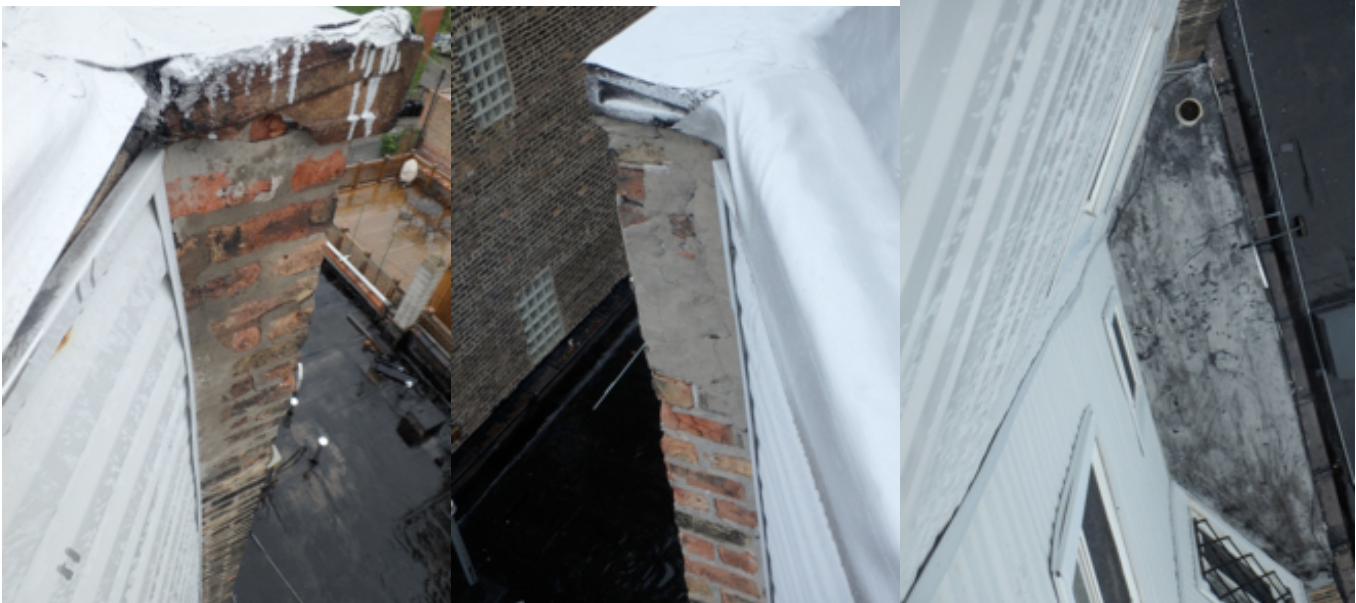
W elevation light well wall and roof views, needs servicing as part of rehab
