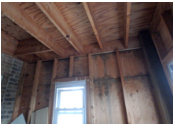
More signs of water intrusion and rot at porch enclosure
