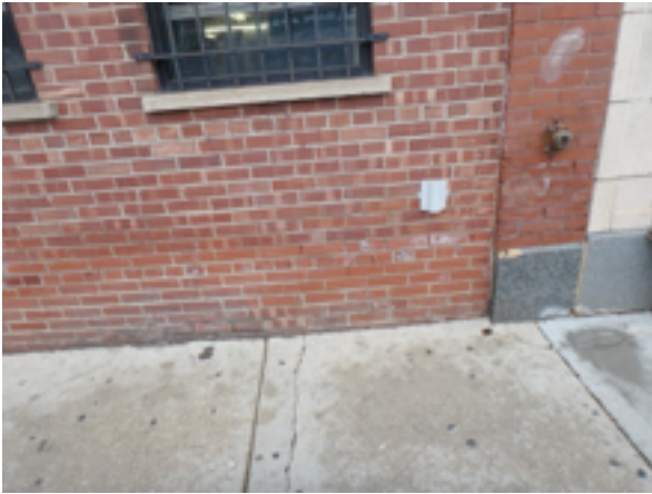
Erosion along bottom of front wall
