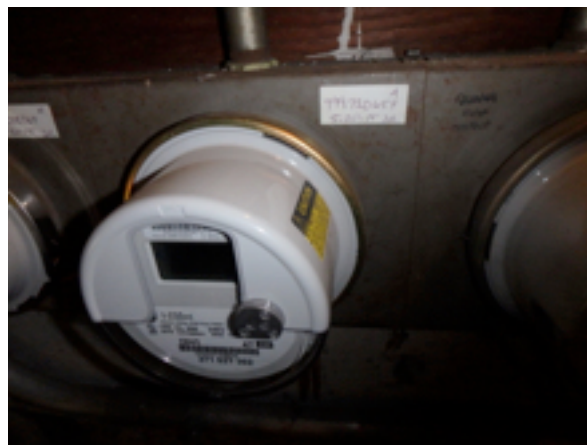
Newer ComEd smart meters installed
