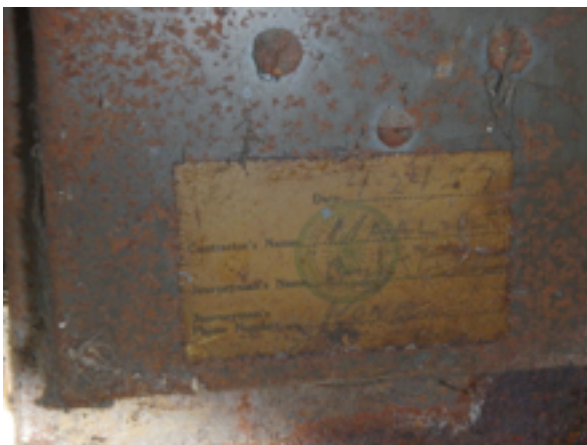
Original installation tag from 1957
